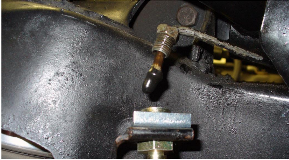
Hose lock location and vinyl cap installed
